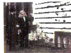
Beverly Richardson points to black water marks on her house. She found out it had a serious mould problem despite an inspection giving it the all clear.
